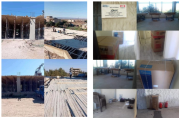
Left: Wadi Khaled’s Community Hall, five weeks after Phase II’s closing date
